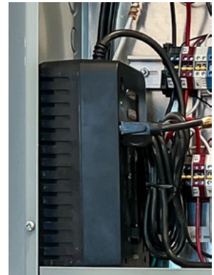
Battery Lowering UPS
